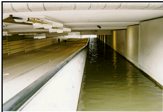
Bicycle/ pedestrian tunnel Utrecht Photo: SWOV, Institute for Road Safety Research, A. Vis
